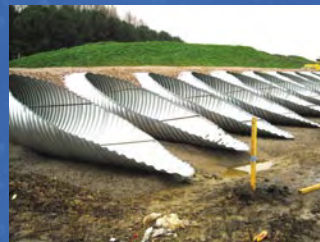
Installation of 30 No x 1500mm Ø Culverts, installed across the Raynesway Flood Plain
